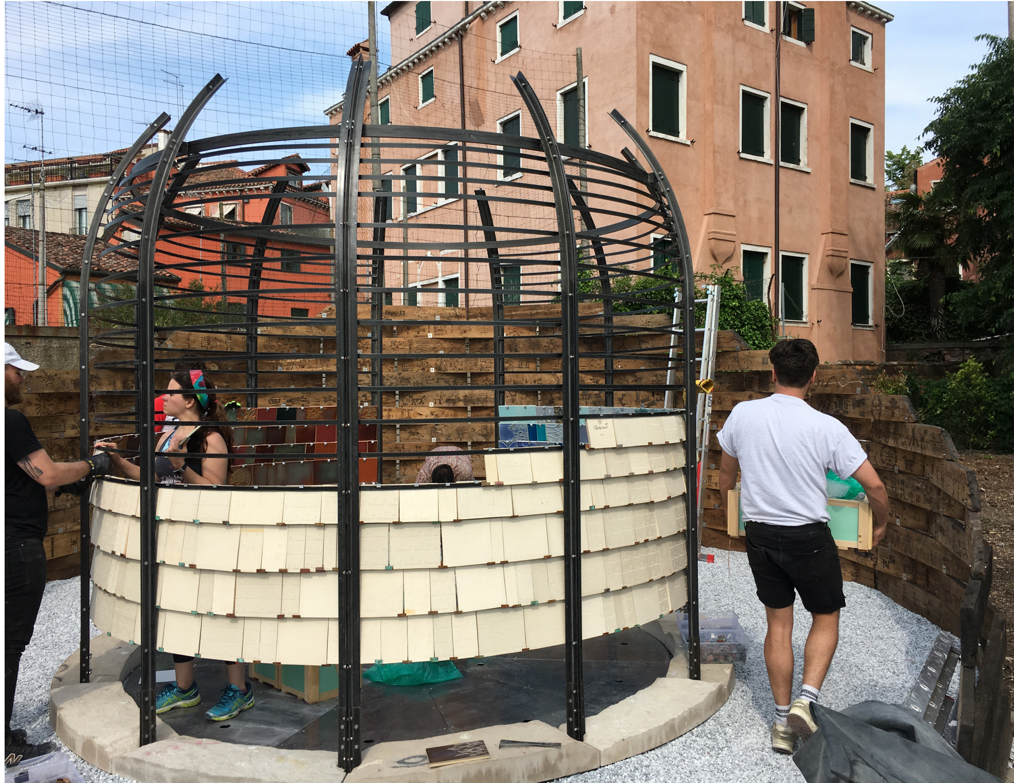
The entire pavilion was constructed on-site in just two short days as a result of our pre-fabricated modular construction.
